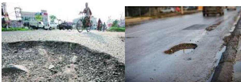
Figure 1: Bad Condition of Road Due to Potholes
