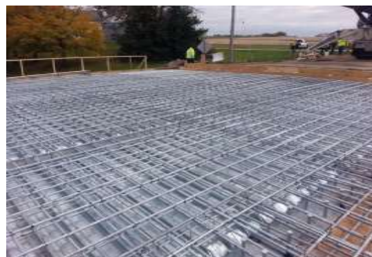
Figure 3: Zinc Coated Reinforcement bars
