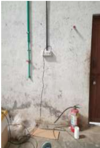
Fire extinguisher was not placed in its proper place
