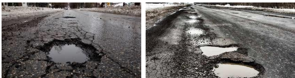
Fig. 1: Pothole crisis all over India
