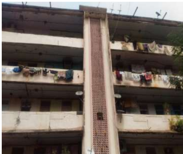
Distressed RCC Findings.
