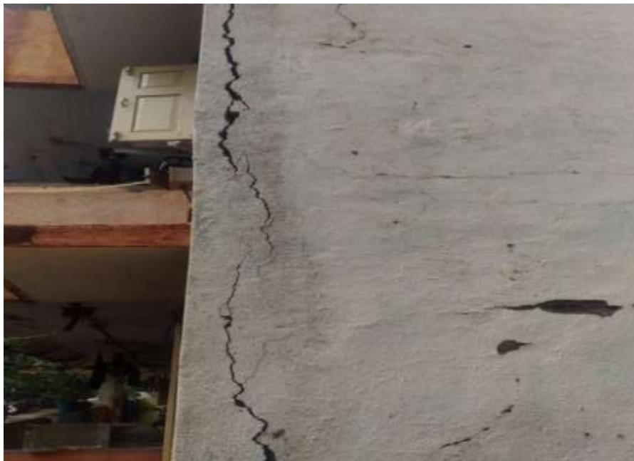
Structural Cracks on the Dead wall.
