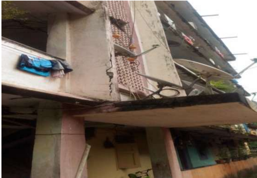
Structural Cracks on the Staircase Passage.
