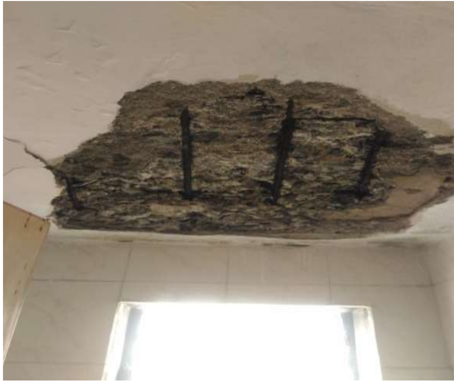
Concrete chipping off from slab exposing reinforcement.
