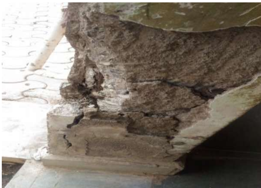
RCC column failure.
