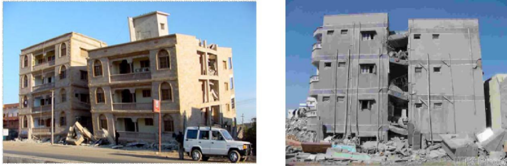
Fig. 2: Failures of OGS building during 2001 Bhuj Earthquake
