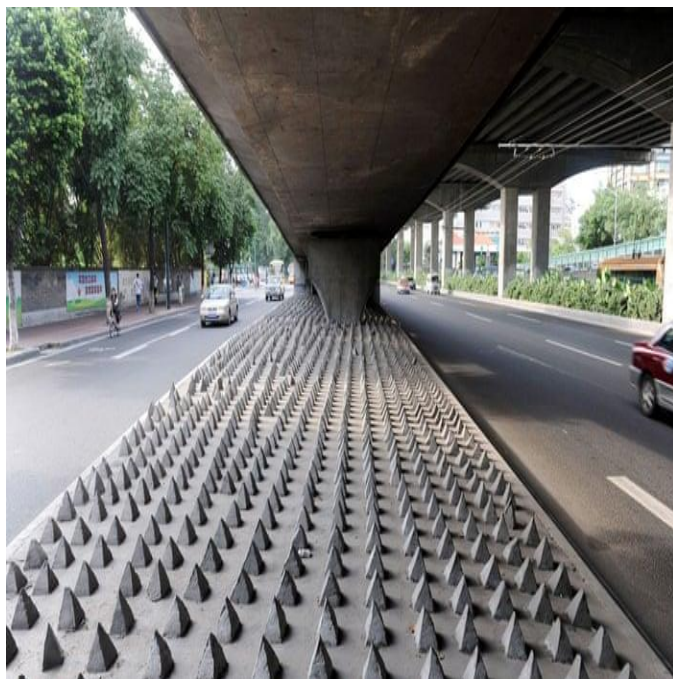
Fig. 2: Concrete spikes under a road bridge in Guangzhou city, Guangdong, China Source: Imagine China/REX
