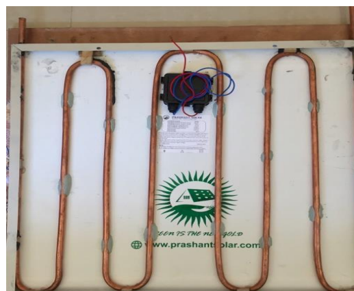
Fig. 5: Installation of the direct heat exchanger at the bottom side of the PV module
