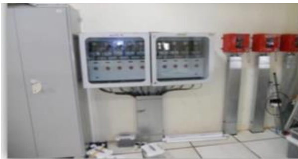
Fig. 2: Fire alarm system control panel in station master room
