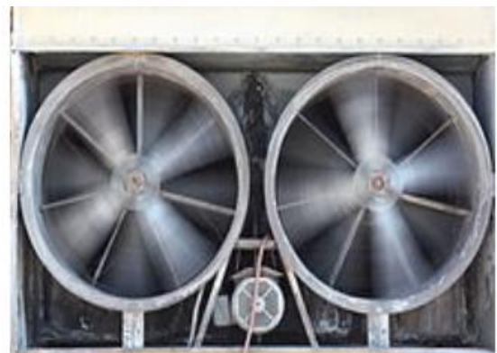
Fig. 1: HVAC ventilation exhaust in the metro station
