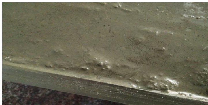
Fig. 6: Hair line cracks
