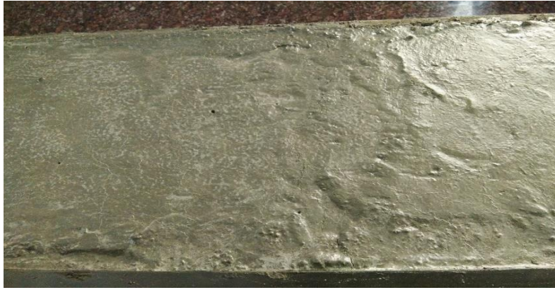
Fig. 8: line full-length crack
