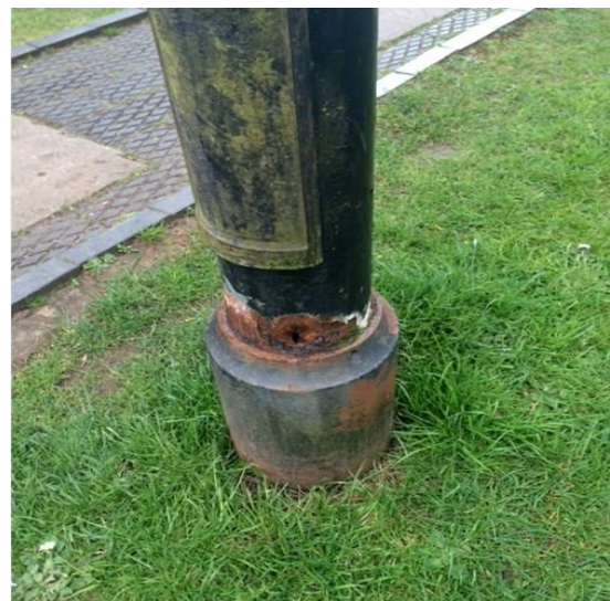
Fig 4: Corrosive street lamp
