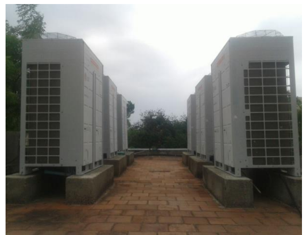
Fig. 2: New LG Chiller ODU at building roof top
