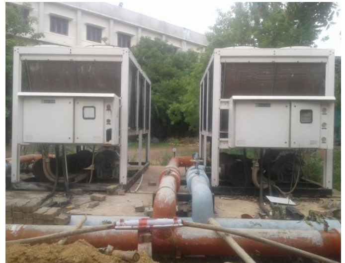
Fig. 3: Old Chiller at building floor level [Disconnected]
