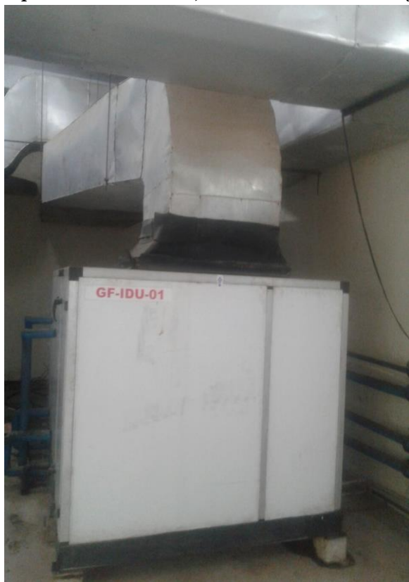
Fig. 4: New indoor unit connected with ODU
