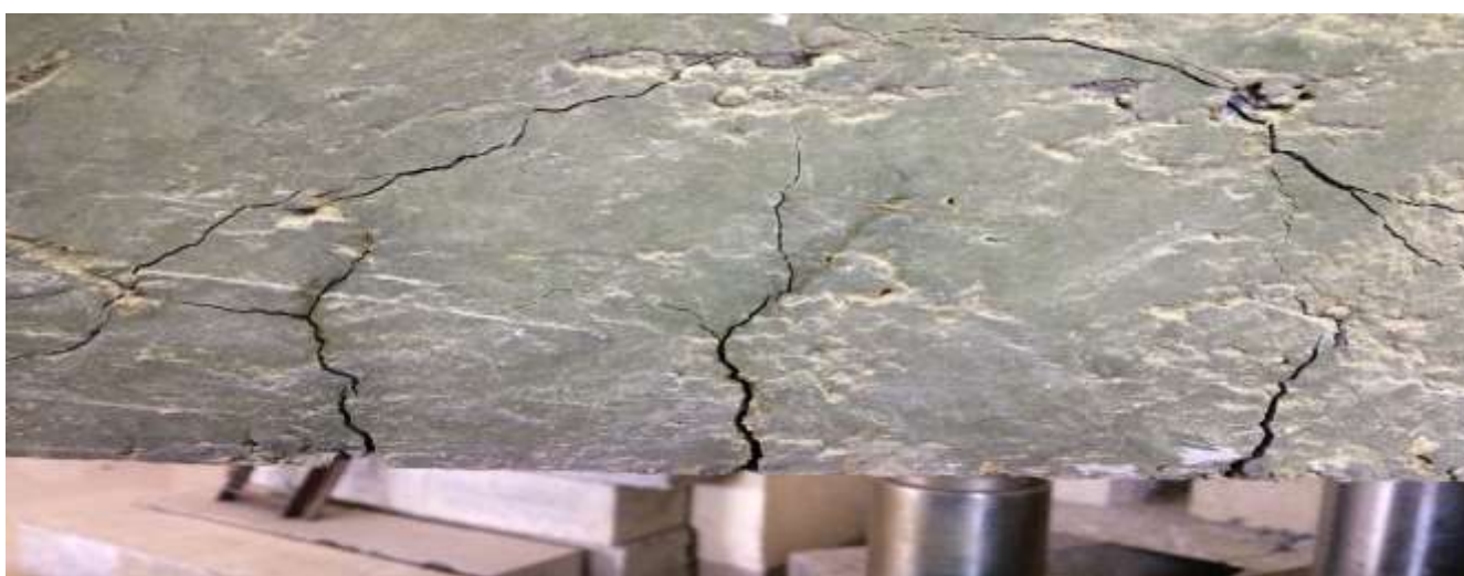
Fig. 3: Cracks development in Flexure (BFRP)
