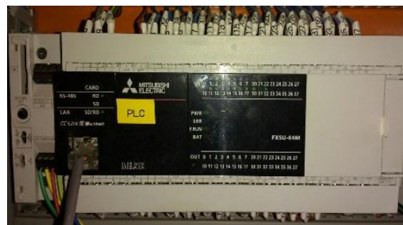
Figure8. Programmable Logic Controller
