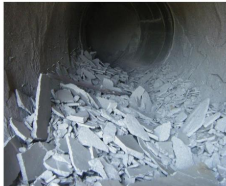
Fig.3 Refractory Failure inside Boiler
