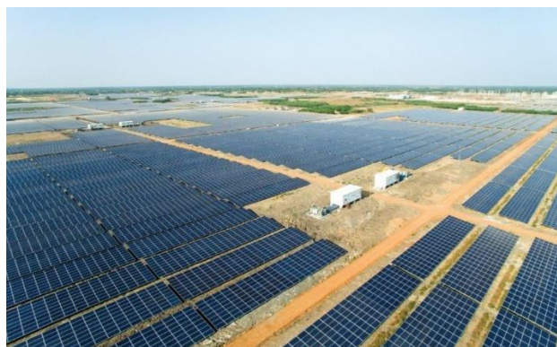
Fig 1 Solar Energy Farm
