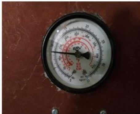
Fig.1 Discharge pressure gauge
