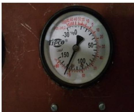
Fig.2 Suction pressure gauge
