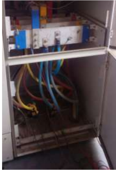
Fig. 2 Live connection to a 22KV/440V panel
