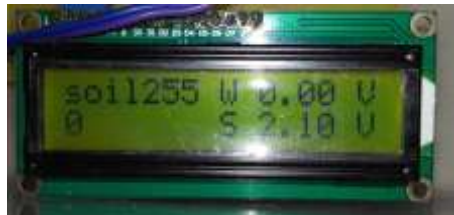
Figure 3. LCD display showing soil moisture value and solar and wind generated voltage.
